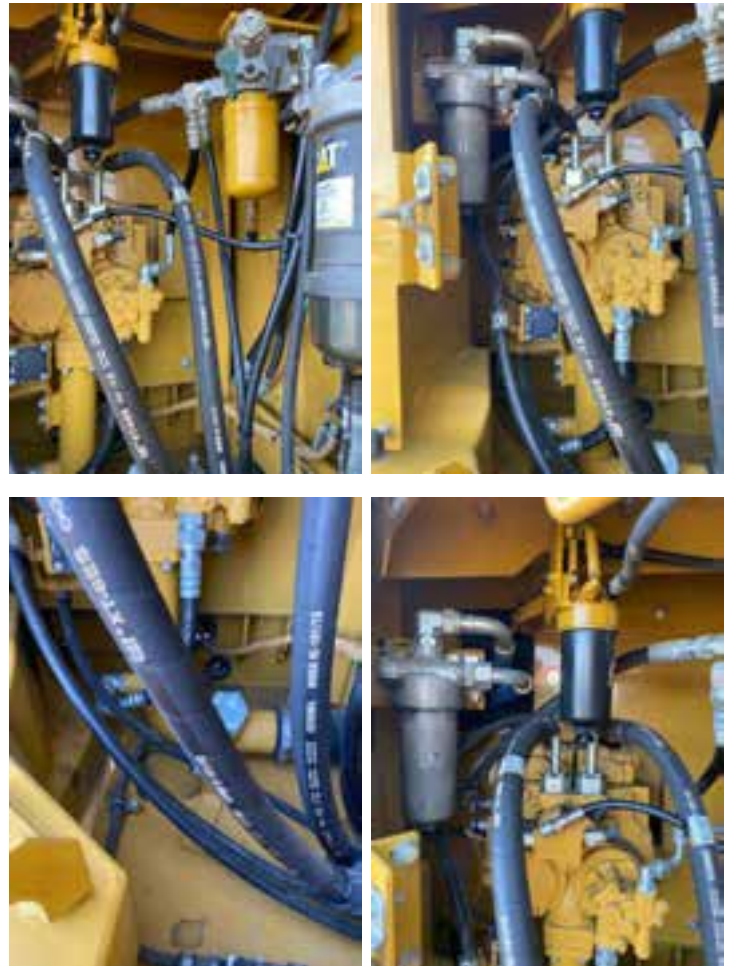
Hydraulic Leaks Photos
